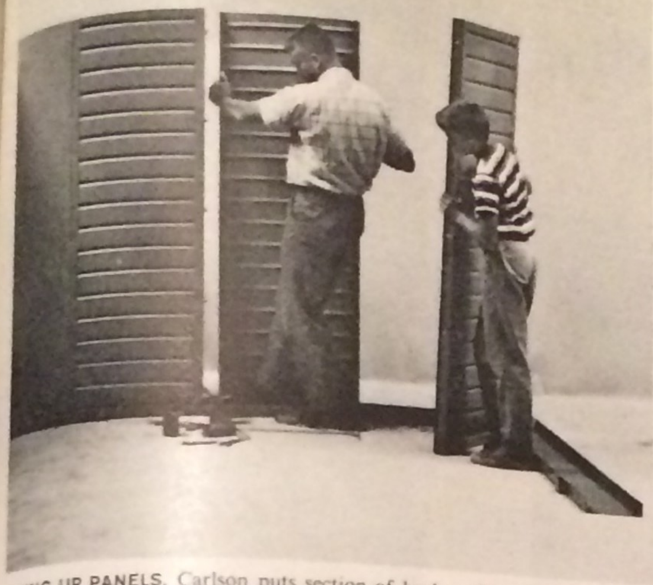
LINING UP PANELS. Carlson puts section of back wall in place as Claude comes up with next piece. The shelter can be erected within four hours by two men using only a screwdriver and a wrench to assemble 73 separate pieces.
